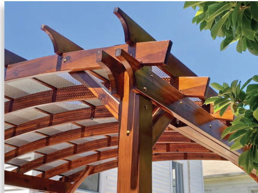
Photo taken 1 year after installation. Photo Courtesy of K. Gates of Oajland, California.
