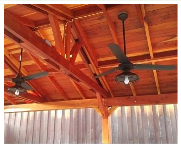
Pavilion with 2 Ceiling Fan Base
