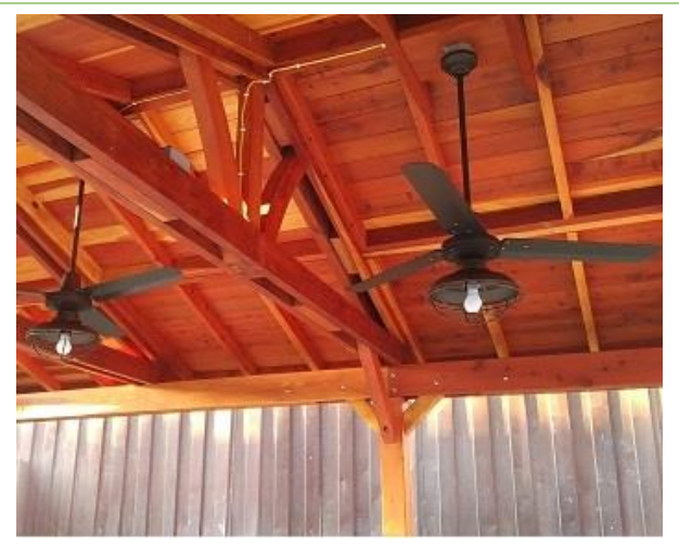
Pavilion with 2 Ceiling Fan Base
